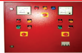
AUTOMATIC FIRE PANEL
